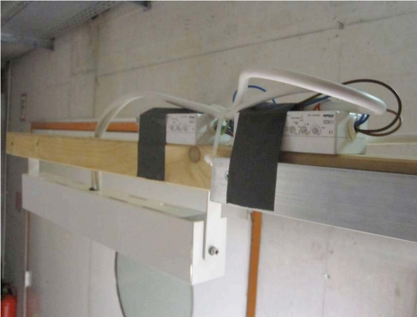
Test of cabling of the wireless actuators with the luminaires.
