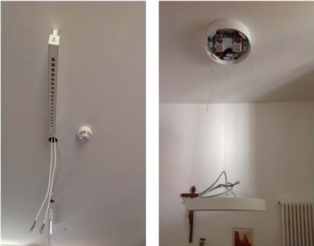
Figure 6: Snapshots from the installation process in one of the test flats of the intervention group. Left: Downlight – Right: pendant light.
